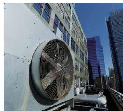
Air conditioning system
